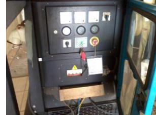
Check main power genset
